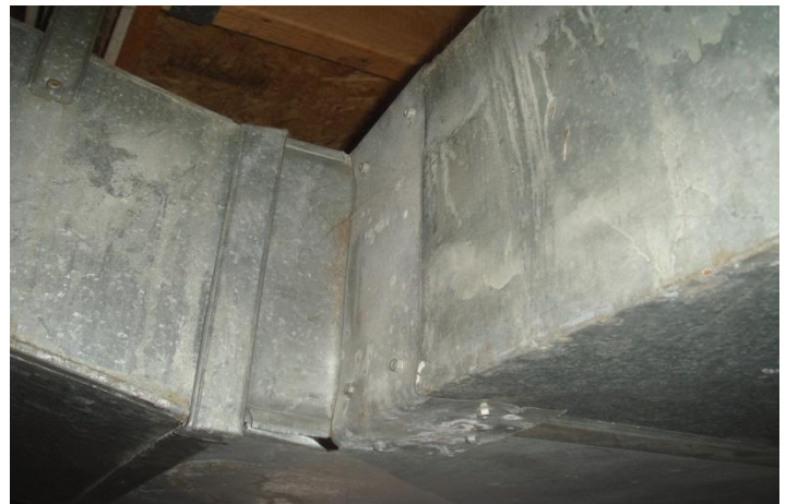
Leaking duct work
